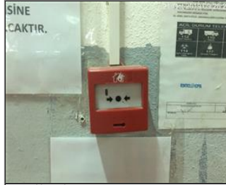
Photo of fire safety equipment Fire alarm button.JPG
