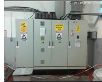
Photo of the inside of the main production hall Electrical panel.JPG
