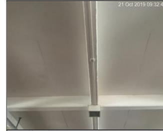
Photo of fire safety equipment Fire early warning system.JPG
